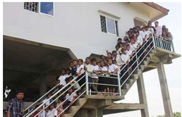
New railing on Mission School provided by CTK after 8 years without one!
